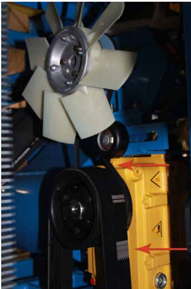
Blower to Pump Belt
